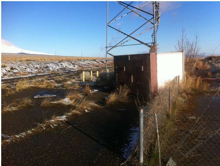
Figure 2.3 Instrument shed at RSLW blown over by high wind.
